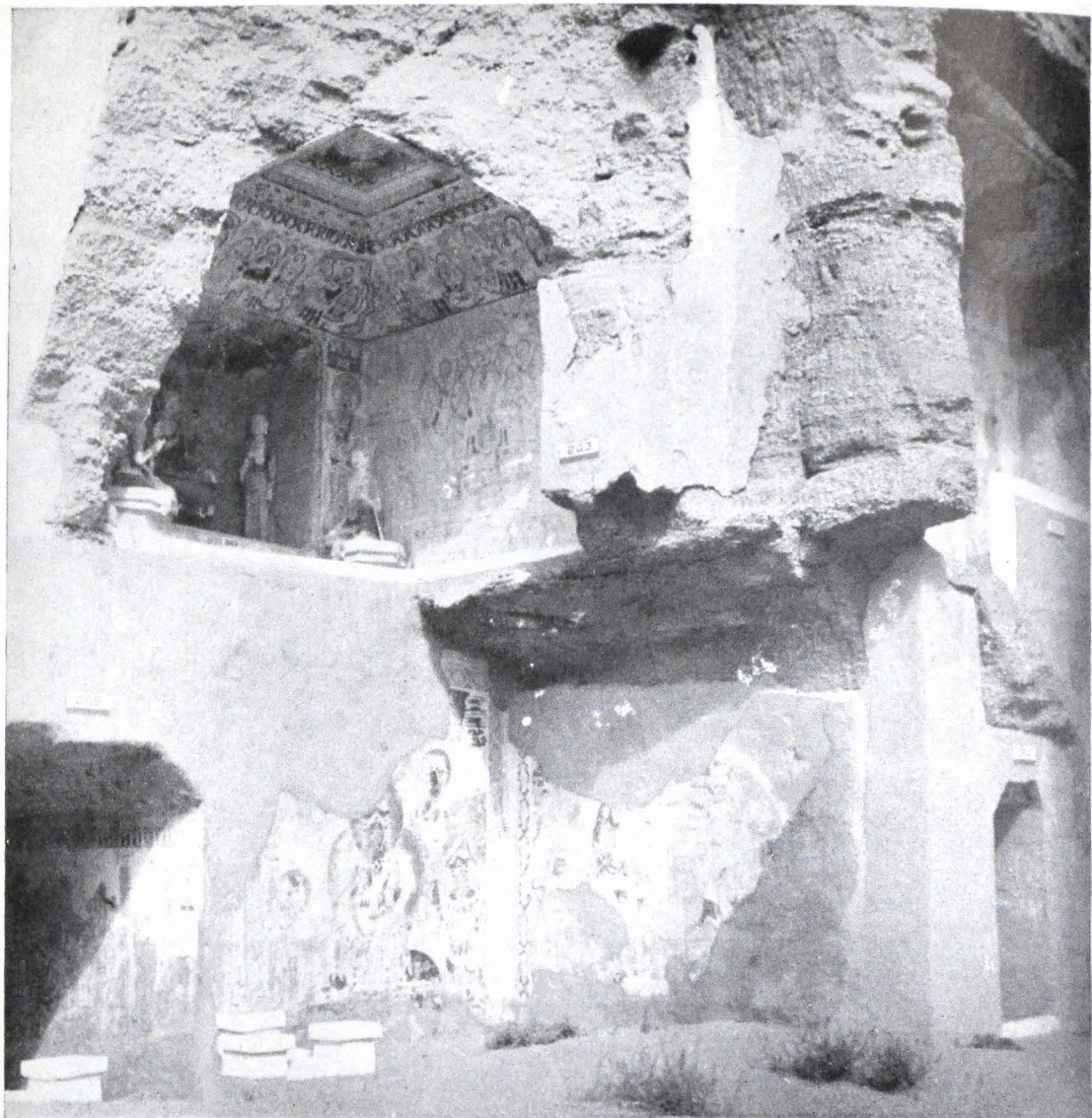
7. Close up of a damaged chapel ( See page 75 ), its shape typical of the majority of chapels both large and small, and even of the inside, about two feet high, of some of the stupas on the east bank of the river bed. The projecting wall at right is all that remains of its ante-chapel. Fragments of wall painting retain some pigment despite decades of exposure to sun
